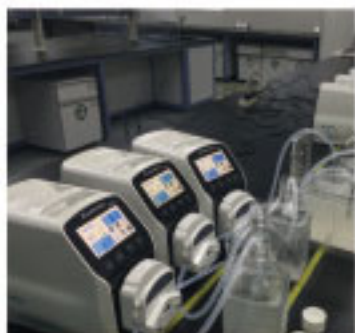
Laboratory chemical dosing
